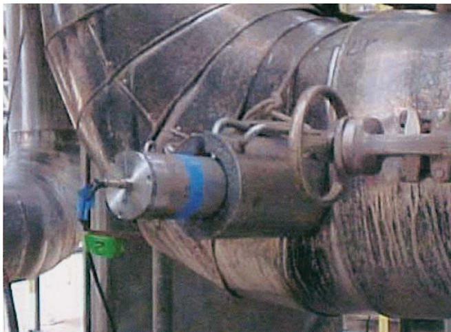
Figure 5 – External detector placement on flow line.
